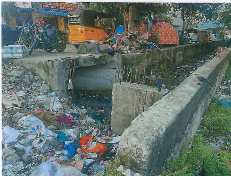
SITE 2 (SEWAGE WATER INLET INTO MEPZ ALONG EAST SIDE BUND OF KADAPERI LAKE)
